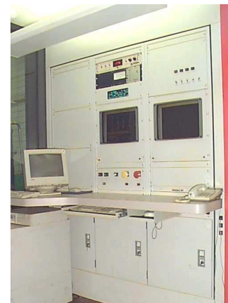
Engine Test Cell Control Panel
